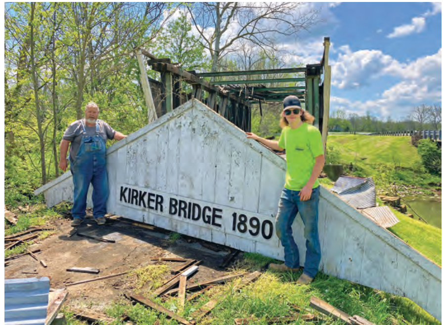
The historic Kirker Covered bridge sustained serious damage in 2024 from a tornado. TOP: Before the tornado. ABOVE: After.
